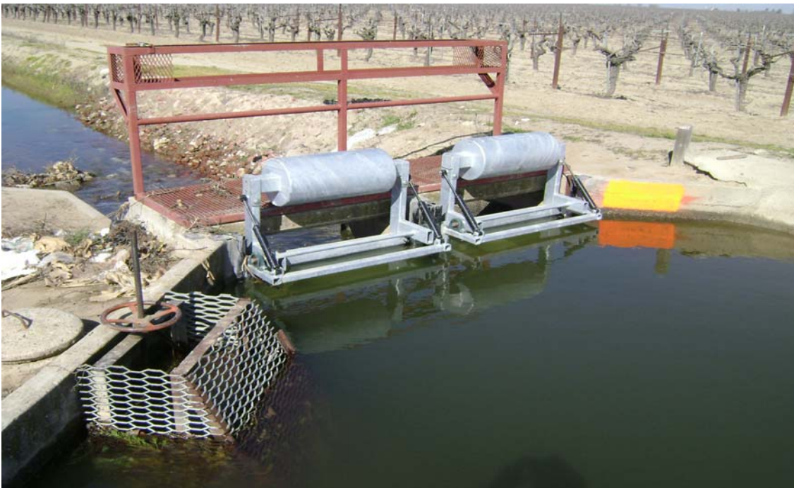
Figure 2. Typical Weir Retrofitted with ITRC Flap Gate
