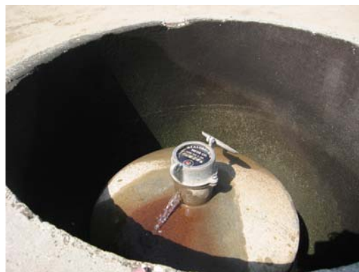
Figure 3. Water Meter at Top of Turnout Riser Located within the Standpipe
