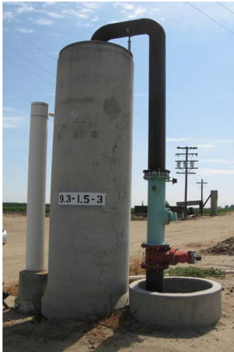
Figure 4. Turnout Riser Located Outside of the Standpipe with Easily Accessible Meter
