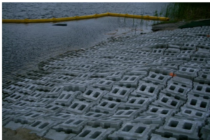
Figure 4. Subgrade Differential Settlement
