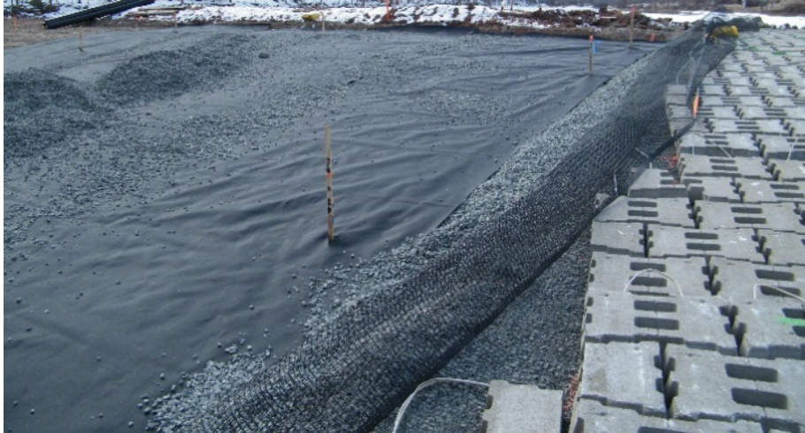
Figure 3. Geotextile Installation Issues
