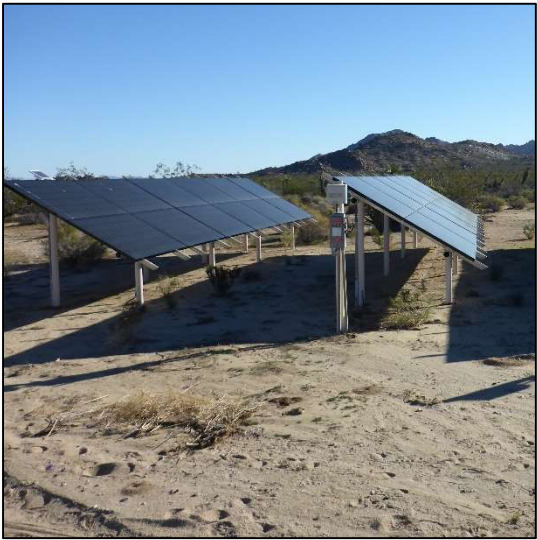
Figure 9-18. Photo of the solar panel farm.
