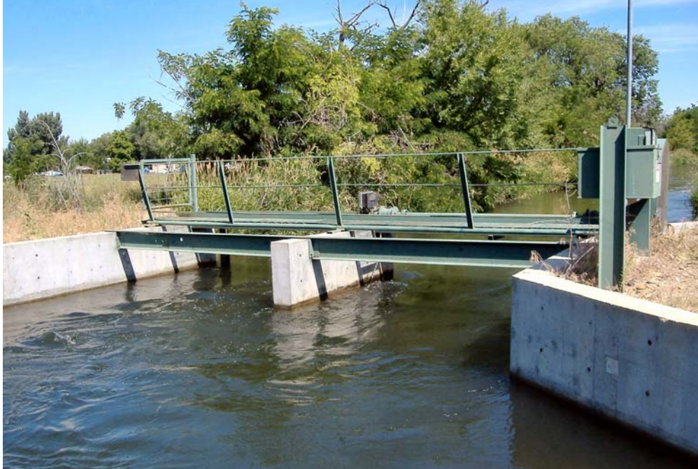
Figure 4. Automated check structure on the Farmers Cooperative Canal. Structure utilizes check boards (left) and automated overshot gate (right) to control water levels.
