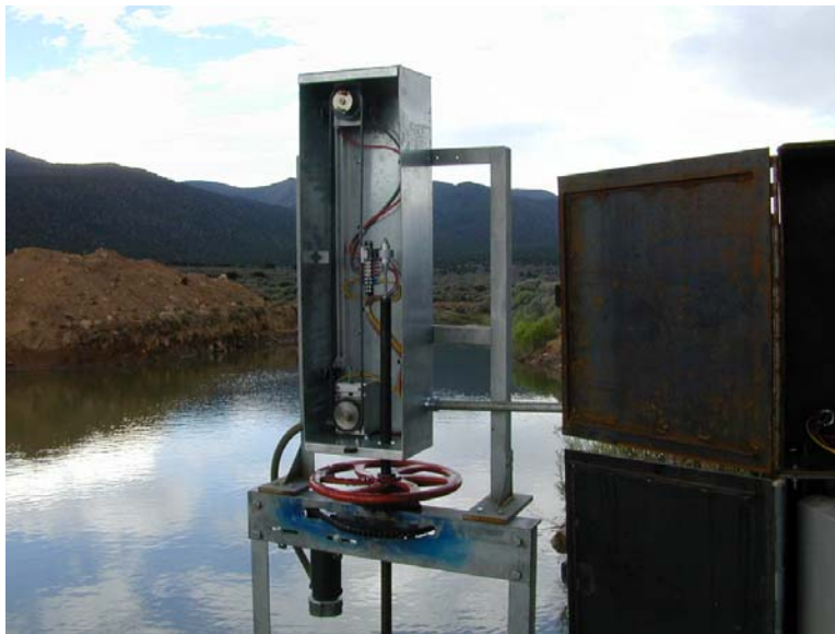
Photograph 3. Gate Actuator Installed on Scipio Canal near Scipio, UT
