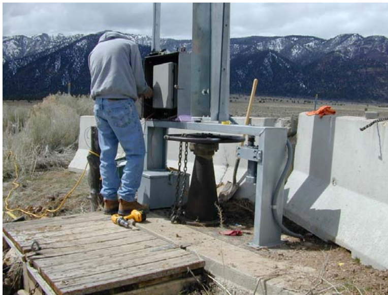
Photograph 4. Gate Actuator Being Installed on a Pedestal Gate on Scipio Dam Outlet Works near Scipio, UT
