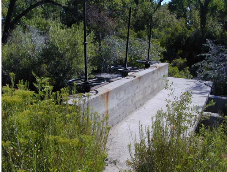
Photograph 1. Huntington Canal Diversion Structure Prior to Gate Actuator Installation near Huntington, UT
