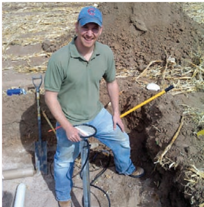
Kendall DeJonge, a graduate student in Civil and Environmental Engineering, installed soil moisture sensing equipment on the Regenes research farm last Spring.
