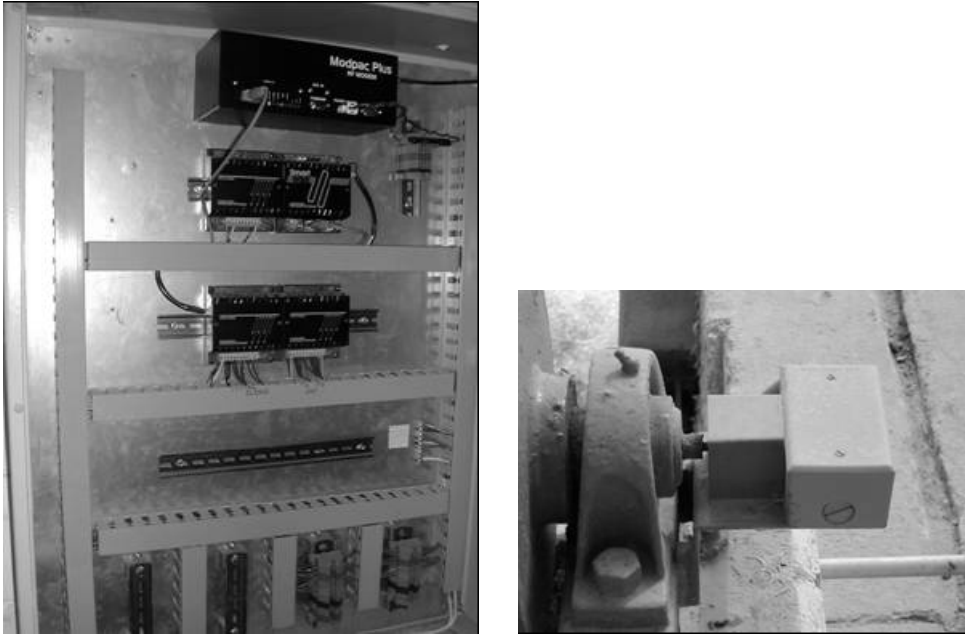
Figure 2. Remote Monitoring System Installed on 2002.
