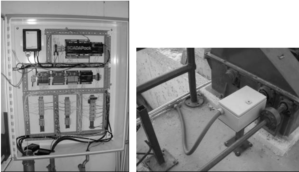
Figure 4. Remote monitoring systems at the KM 4+100 Control Structure.
