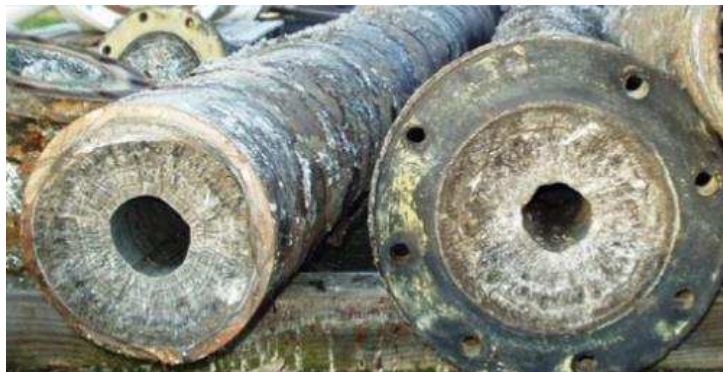
Figure 7- Accumulated struvite formation in WWT pipes (Suszyński, 2016)
