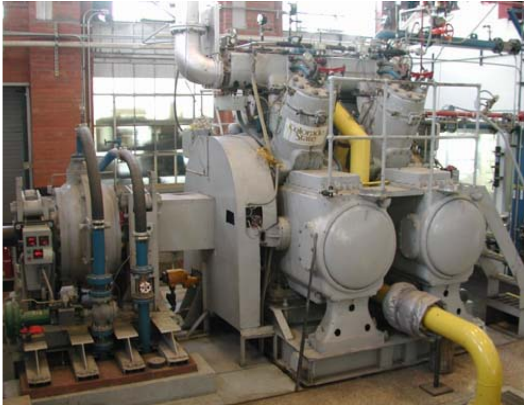
Figure 2.1 - Cooper Bessemer GMV-4TF
