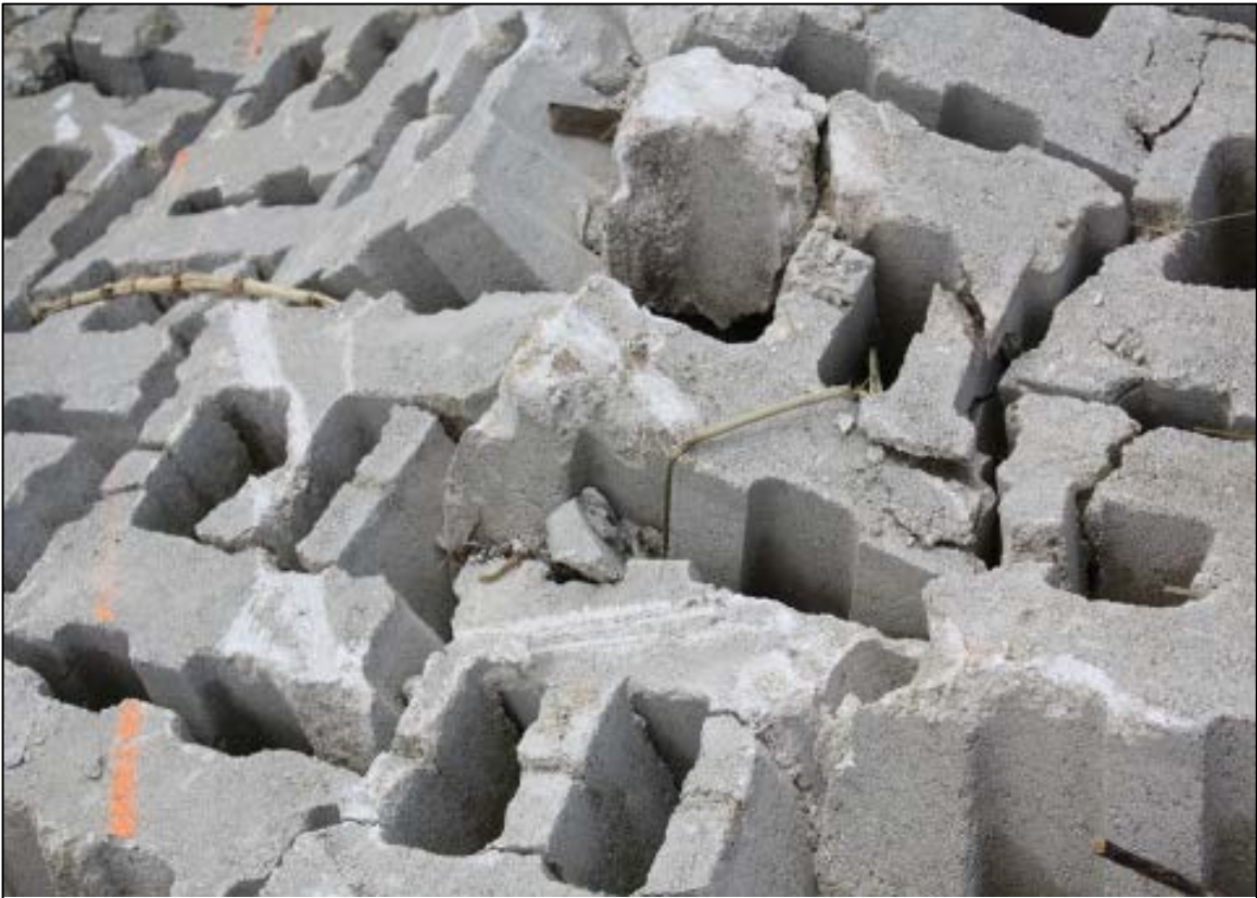
Figure 10. ACB Armoring on Portugués Cofferdam Damaged from Debris Impact (Concrete Jersey Barriers and Concrete Slabs).
