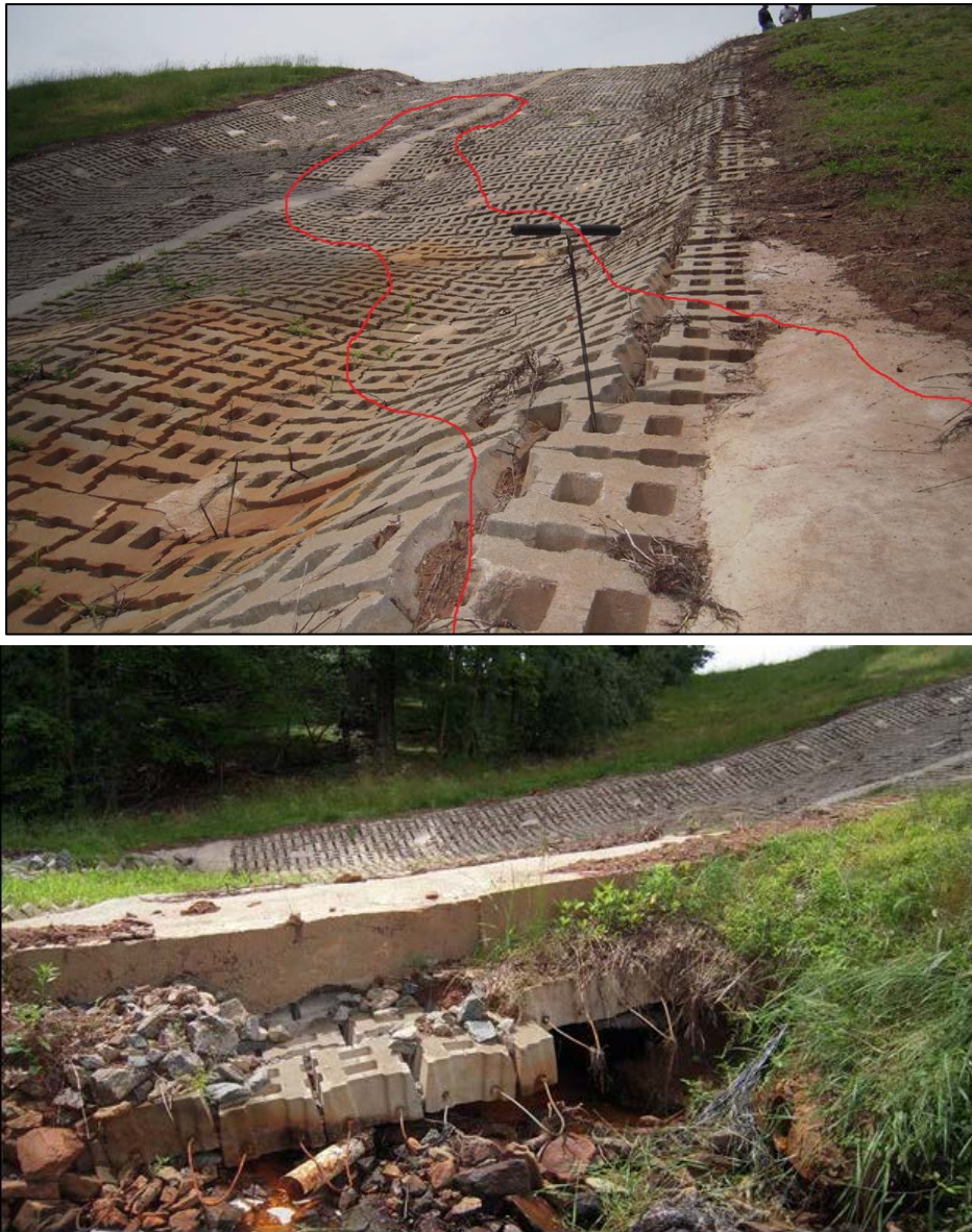
Figure 8. Photographs Showing Piping Under the ACB Armoring Over an Embankment (Top) and the Piping Outlet (Bottom).
