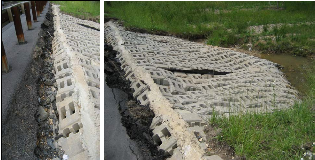
Figure 18. Photographs of ACB Installation at Grover's Mill Dam Showing Armoring Units Damaged from Inadequate Transition Details at the Top of the Installation
