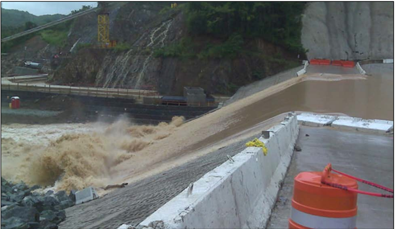
Figure 4. Photos Showing Overtopping of Portugués Cofferdam during Significant Overtopping Event (Photos Courtesy of Jacksonville District USACE)
