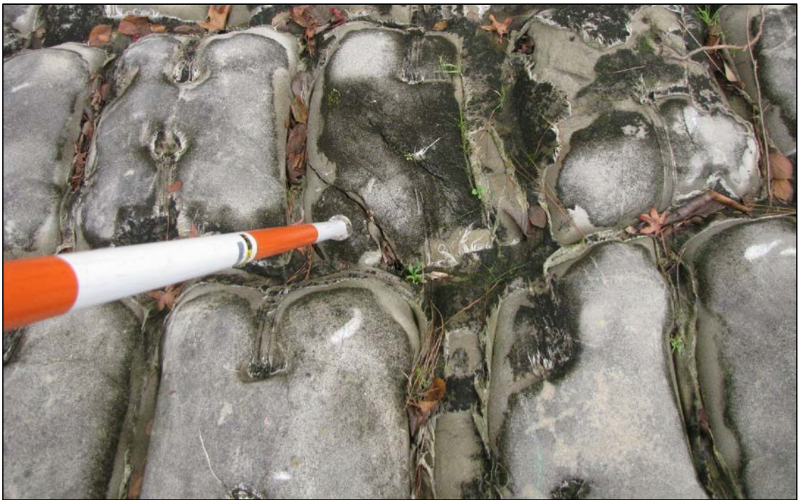
Figure 15. Photographs Taken in 2015 Following a Overtopping of Forest Lake Dam during Hurricane Joaquin Showing Condition of Fabriform ACB System Installed in the 1980s
