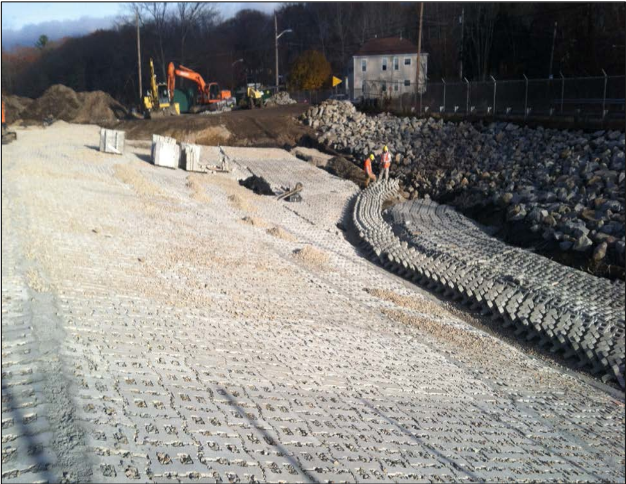
Figure 16. Photograph of ACB System with Armoring Units Installed at the Toe of the System to Provide Energy Dissipation of the Flow
