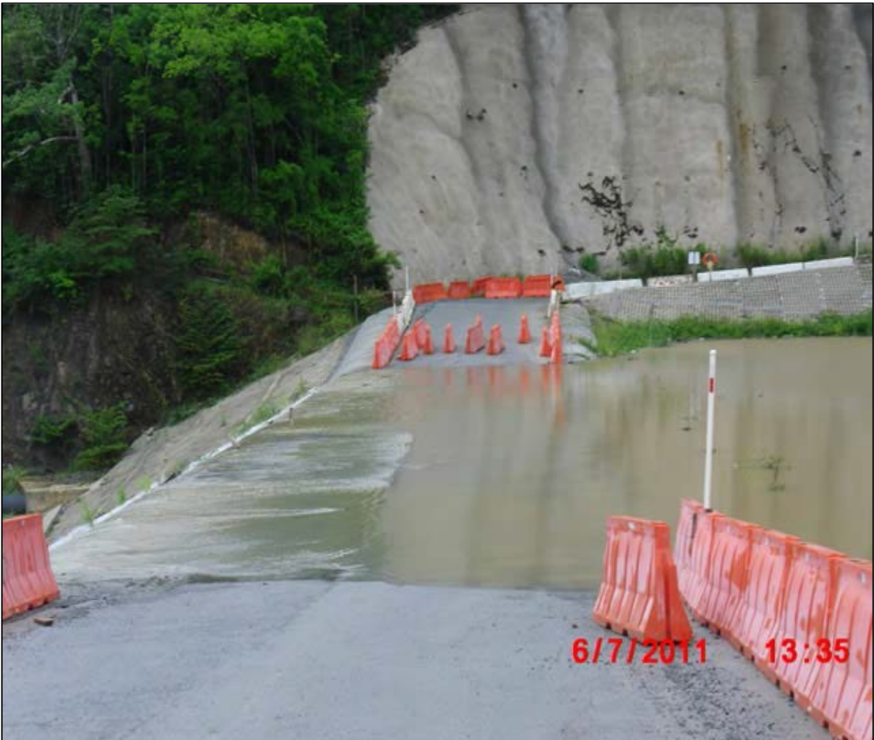
Figure 11. Photograph showing plastic jersey barriers used to replace the concrete jersey barriers at Portugués Dam to prevent impact damage to the downstream ACB armoring should the jersey barriers become unstable and wash down the downstream face of the ACB armored cofferdam.
