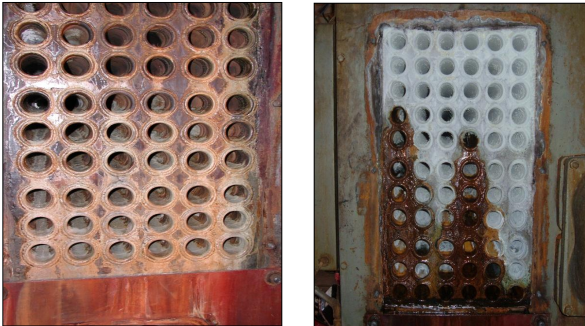
Figure 3-1 Picture of the Fire Tube in June 2010 (to left) and in March 2011 (to right)
