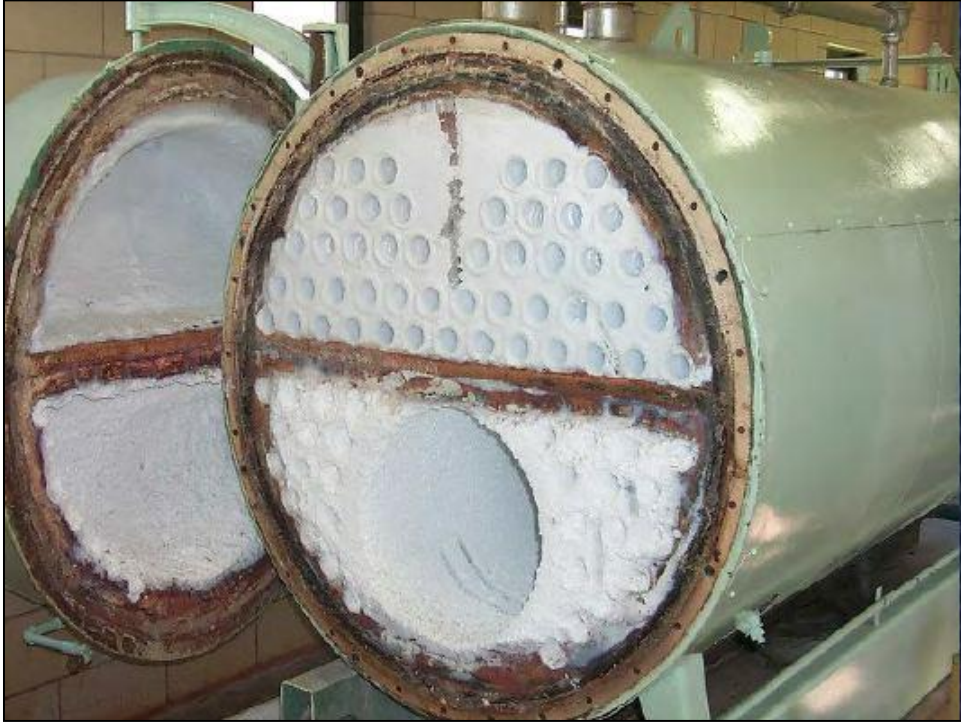
Figure 2-4 Siloxane Deposition in a boiler
