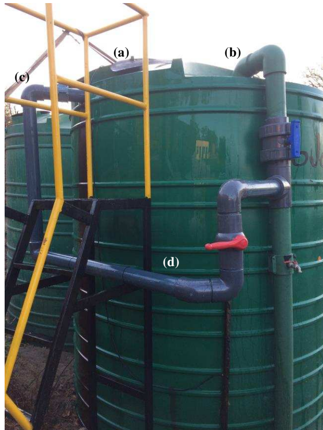
Figure 3.3: Photograph of Tank 2 with external modification; (a) access point, (b) original vertical inlet, (c) new horizontal inlet, (d) external modification
