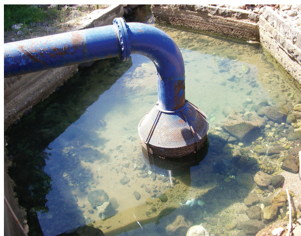
Wazzani Pumping Station
