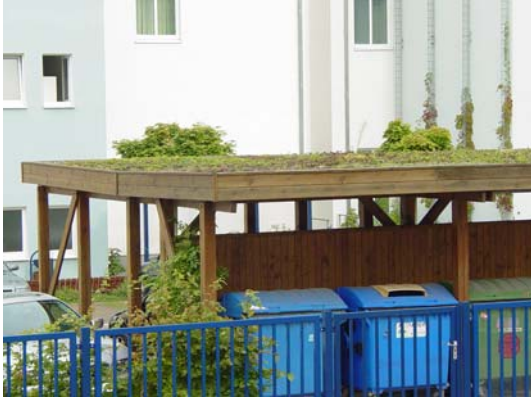
Figure 4.29 Green Roof Shed. Green roofs are installed on refuse sheds in Rostock, Germany to retain rainwater and reduce the “rain tax” Germans pay for storm water runoff. This roof is located a short distance from the WIRO roof.
