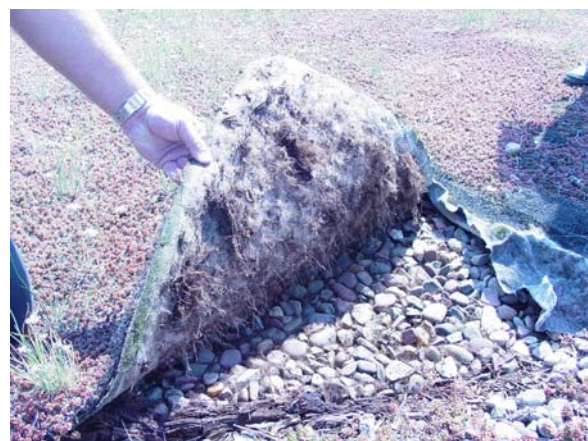
Figure 4.20 Building 3. Only sedums remain on the portions of the roof with only gravel and no soil.
