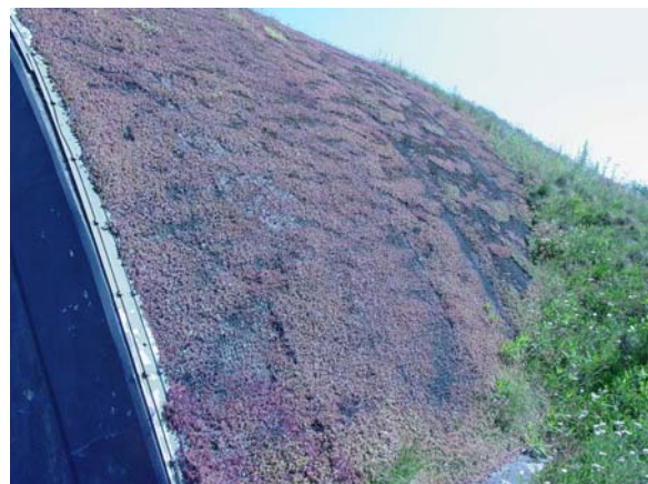
Figure 4.16 Bunker 1. The plastic sling/coil that holds the mats in place can be seen through the sparse vegetation.
