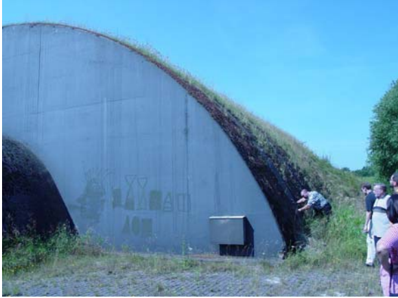
Figure 4.13 Bunker 1. Signs of neglect are evident.
