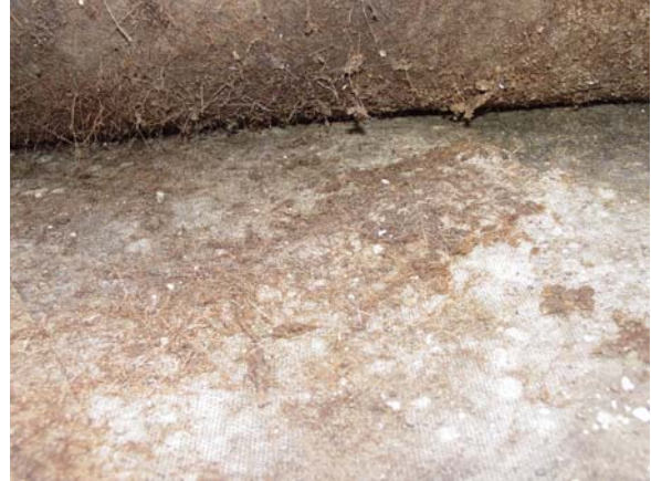
Figure 4.28 WIRO GmbH Roof. Slender sedum roots can be seen on the bottom of the vegetated mats and broken off on the Famogreen Ret membrane underneath the mats. Roots grow through the white fabric to reach the water retaining gel crystals below.
