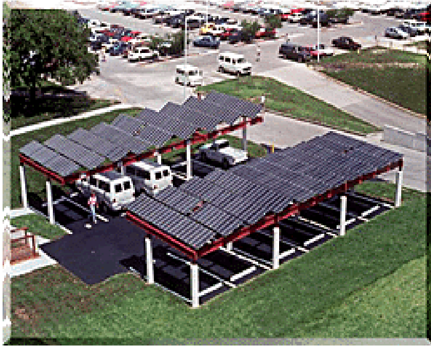
Figure 10. Photovoltaic Panels over Parking Lots
