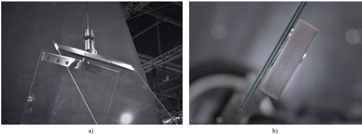
Fig. 12 a) Pivot detail with frictionless rotation and swinging ability, b) One-sided eccentric bracket detail (© DefineEngineers / seele).
