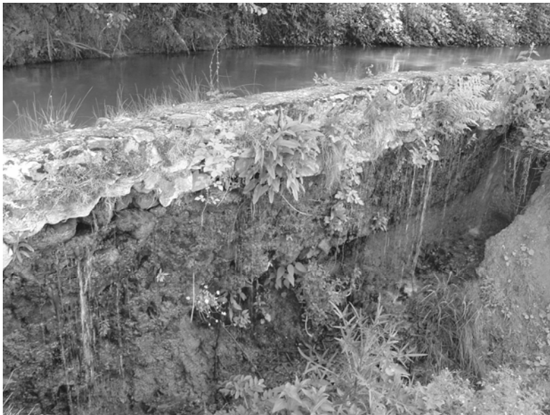
Fig.2. Deteriorate sector of supply channel MHC1
