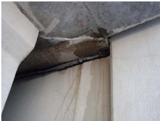
(a) Deck cracking
