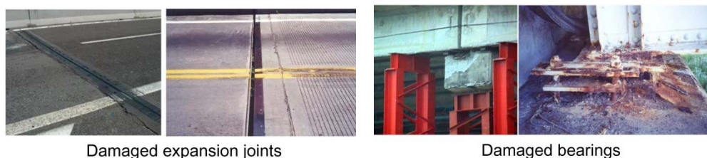
Fig. 3 Typical failure modes of expansion joints and bearings
