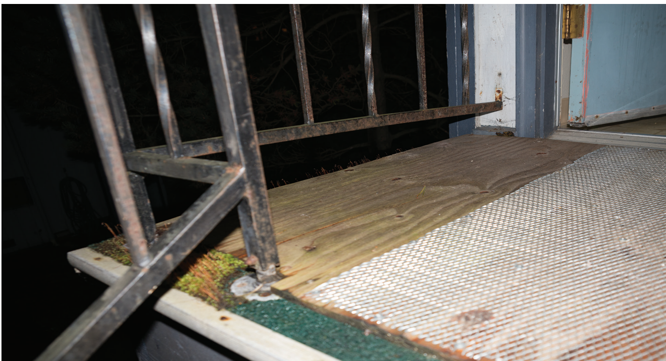
Wood rot outside of Porché Reith’s home. | Jessica Ernst
