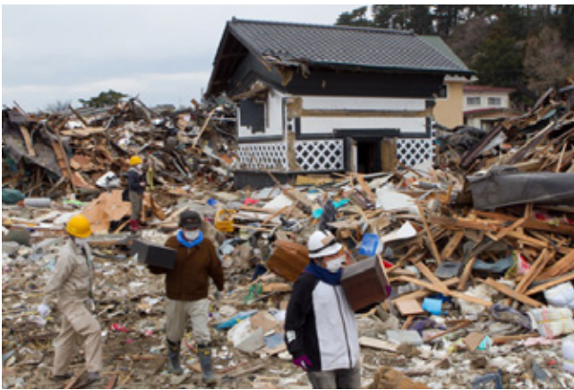
Fig. 5.4 Salvage Operations of Honma Family Historical Materials (Ishinomaki city, Miyagi Prefecture, Apr.6,2011)
