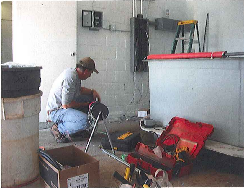
New circuit panel boxes were installed to provide power for water handling needs.
