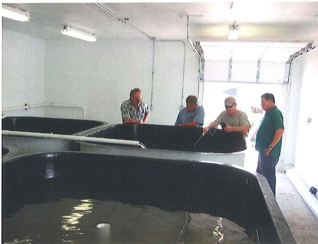
Four tanks were installed in a bright room whose walls could be washed.
