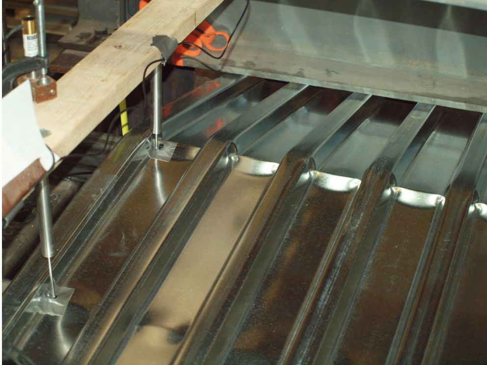
Figure 48: 18 Gage Deck Positive Bending - Further Buckling.
