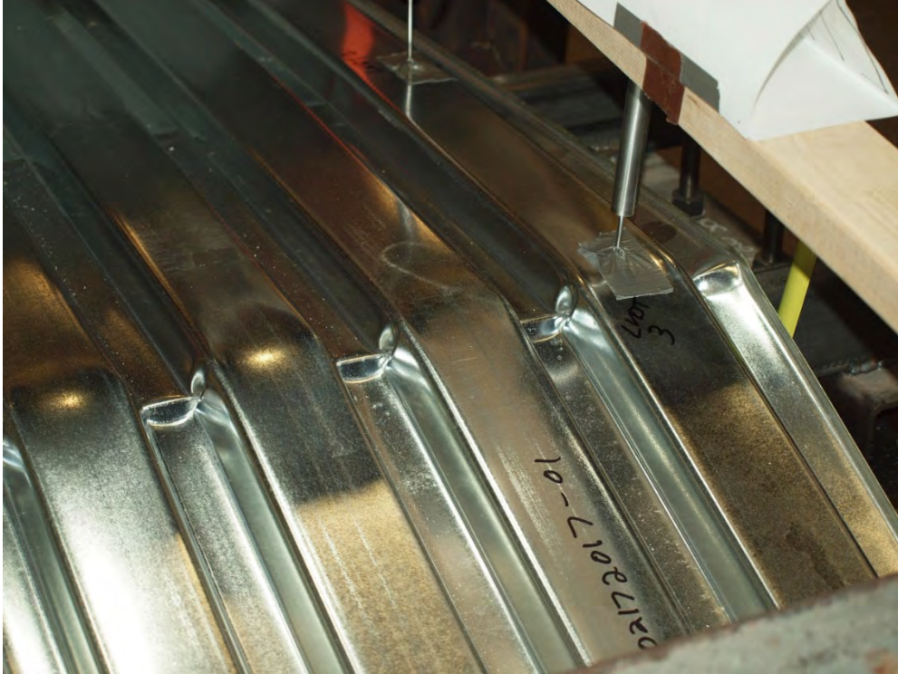
Figure 40: 18 Gage Deck Negative Bending - Further Buckling.
