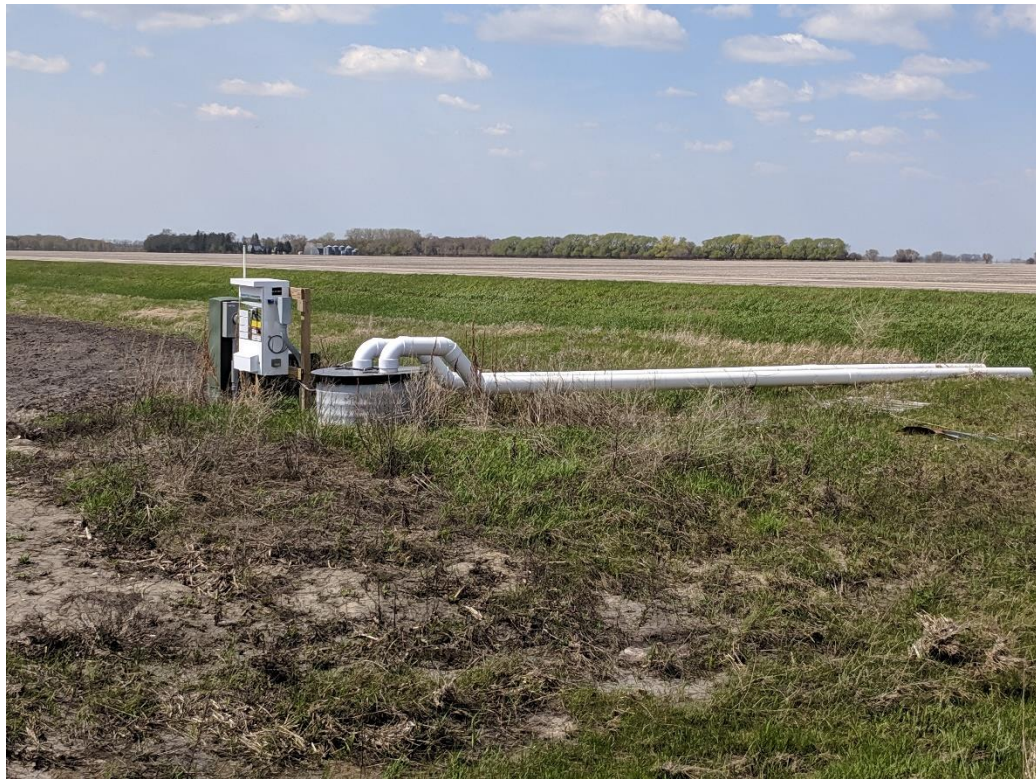
Figure 3. Controlled drainage system in in ESTER Township, Polk County, MN, on May 13, 2019 (Photo taken by the Author).
