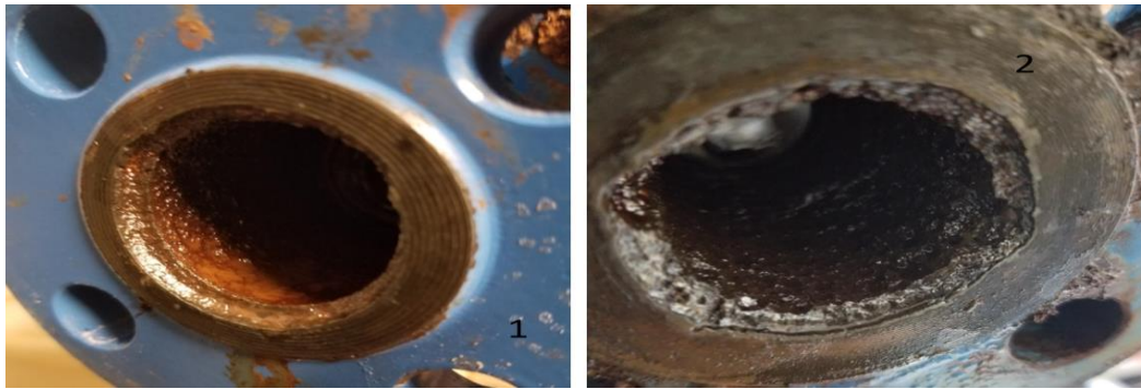
Figure 45. Valve corroded internal view.
