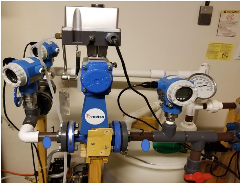
Figure 36. Interconnecting piping with visible oxides.
