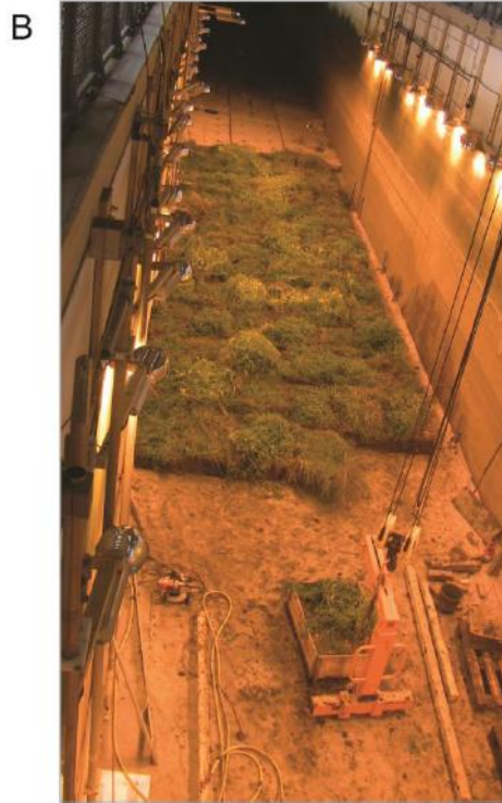
Figure 1: A: Experimental test-section in the Large Wave Flume (Grosser Wellenkanal, GWK) showing platform positions (1-6) for surface elevation measurements; B: view of the vegetated test section at the mid-point in construction, (see text for details), looking towards the wave paddle (photo: I Möller)
