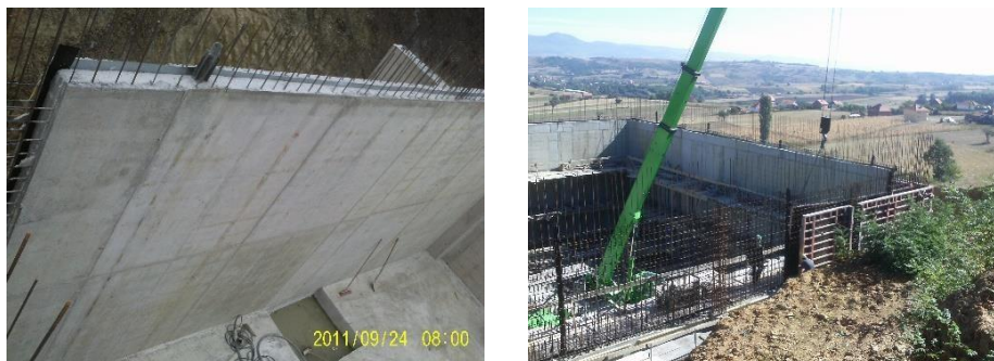
Figure 2: Images from practical application of joint tubes for induction of cracks in concrete wall
