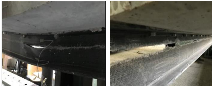
Figure 14. Failure of hybrid beam (cracking in concrete and inter-laminar shear failure)
