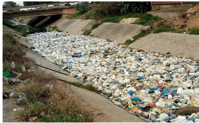
Figure 2. Drain Choked with Plastic Waste
