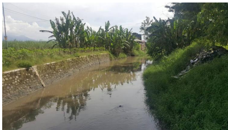
Figure 1. Condition of the Afvoer Sidokare River
