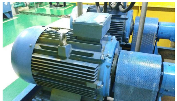
Gambar 7 Cooling Water Pump
