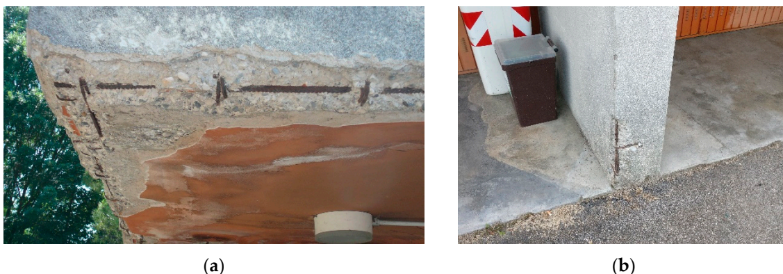
Figure 8. Maintenance status of the building. (a) Concrete cover detachments in the walkaway beams. (b) Concrete cover detachments in partition walls.
