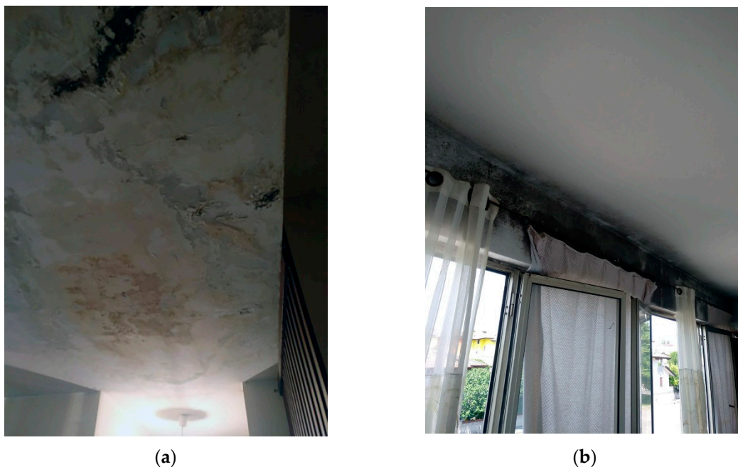
Figure 6. Maintenance status of the building (a) Rainwater infiltration problems causing blooming in the plaster. (b) Moisture patches in the most exposed walls.
