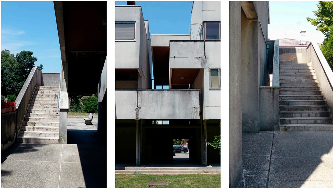
Figure 3. From left to right: western, central and eastern stairwells leading to the external walkways.
