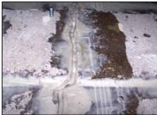
Figure 2.4 Cracks of Upper Stillwater RCC Dam (Smoak 1991)
