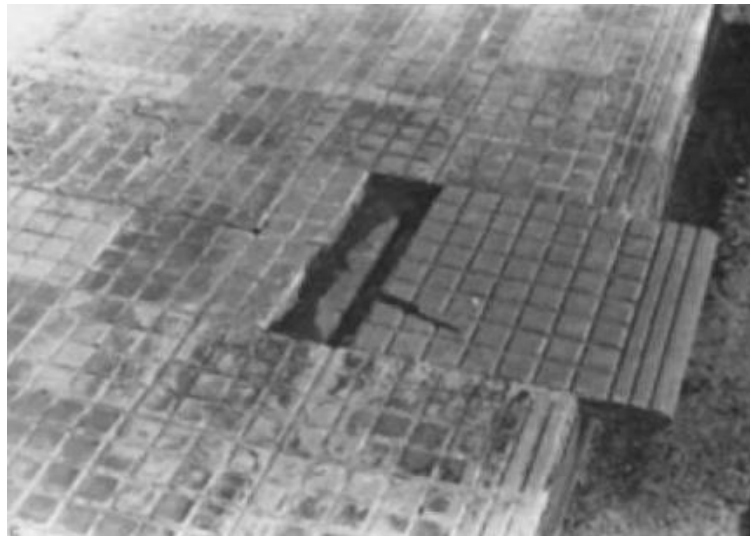
Figure 2.3 Movement of the unfixed tiles on the span of the Koyna Dam (Gupta 1992)
