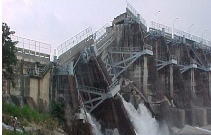
Figure 2.2 Shih-Kang Spillway Weir Destroyed Spillway Units (Sugimura, 2001)
