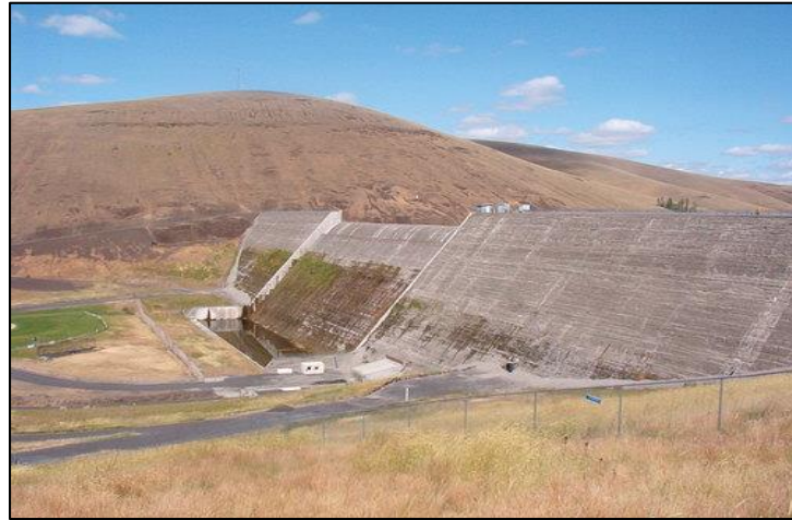
Figure 2.5 Willow Creek Dam deformed face with seepage (Smoak, 1991)
