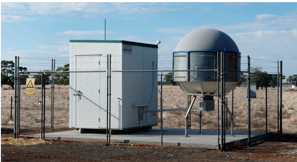
Figure 1. IMRU equipment cabin and antenna, Hay, New South Wales (NSW), April 2017.
