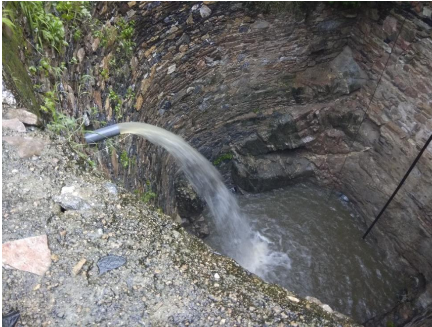
Figure 3. Runoff discharge into well after it was collected in the pit and had passed through the filter.
