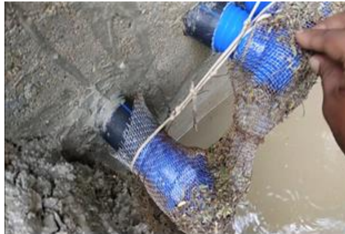
Figure 9. Recharge pit with filters. and clogging of the flow meter inlet.
