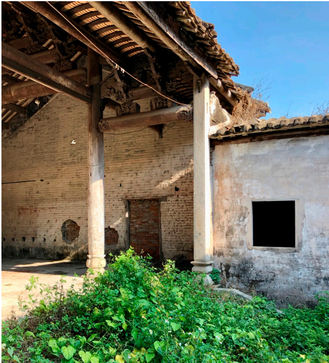
Figure 3. A deserted temple building in Wushi village (Zhongshan Prefecture, southeast China), used as a factory during the Mao era, is subject to a fund-raising campaign for its restoration. Photo by Denis Byrne, 2018.
