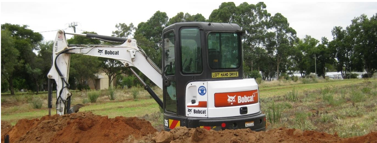
Figure A.2: Backhoe loader used for digging the two adjacent trenches for the field experiment.
