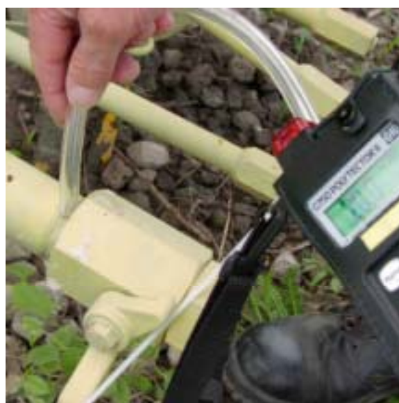
Photo 8: Valve screening with GfG-unit.
