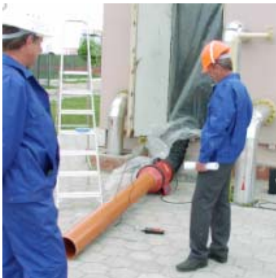
Photo 9: Volume measurement at a fuel gas preparation unit. Kursk, May 2003.
