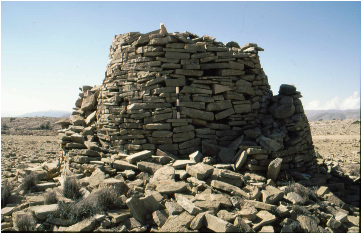
Fig. 6. Tower tomb Shi8 shows the construction of an inner wall and a facade.
