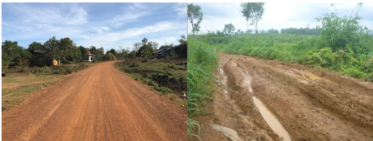
Figure 8: Examples of roads in Keo Seima Wildlife Sanctuary in good (left) and bad (right) condition.
