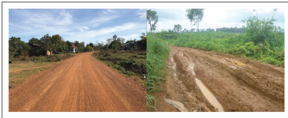
Figure 2. Examples of roads in Keo Seima Wildlife Sanctuary in good (left) and bad (right) condition.
