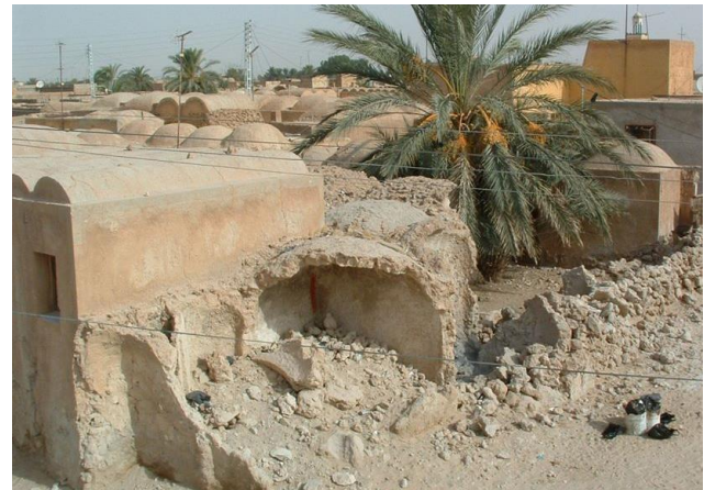
Figure 4. The degradation states of building in the Guemar.
