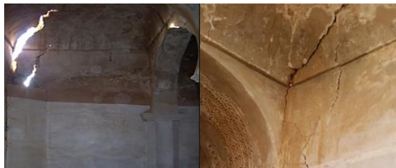
Figure 6. Fractures at the corners of the domes, along the diagonal arches.
