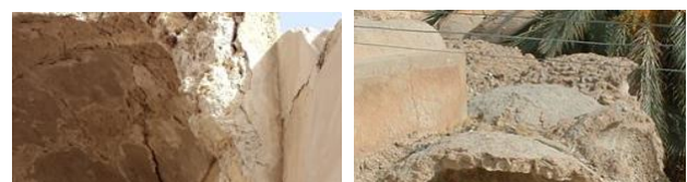
Figure 5. Crumbling of the surface layers of plaster.
