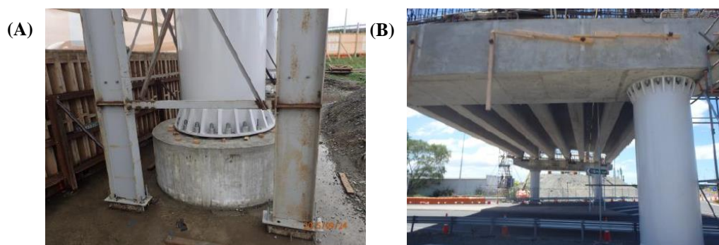
Fig. 2-2 View of the low-damage connection installed at the (A) bottom and (B) top surfaces of the rocking piers in the Wigram-Magdala Link Bridge, New Zealand. ( figure taken from Routledge et al. 2016 )
