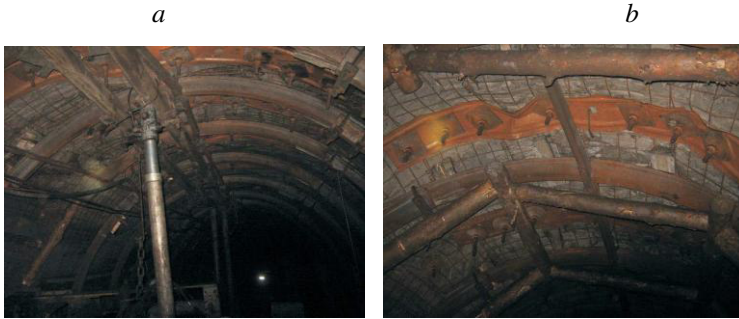
Fig. 14. Condition of the roadway 585 of the Yubileynaya Mine: a - 10 m to face end; b - 60 m after the face
