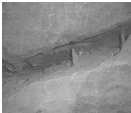
Fig. 4. Horizontal reinforcement and corrosion of reinforcement in the wall of the base F-3
