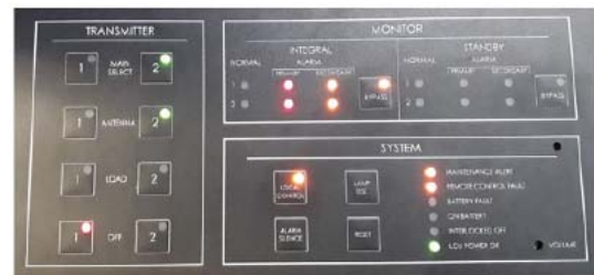
Fig. 1. VOR SELEX Built-in Monitor [4]
