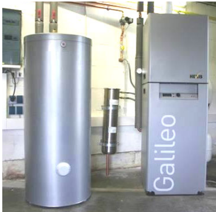
Figure 1: Galileo 1000 with domestic hot water tank in a single-family home.
