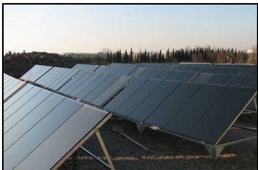
Figure 2a: PV panels.
