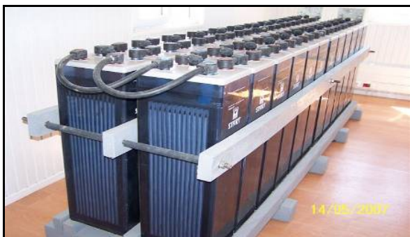
Figure 3a: Lead acid batteries.
