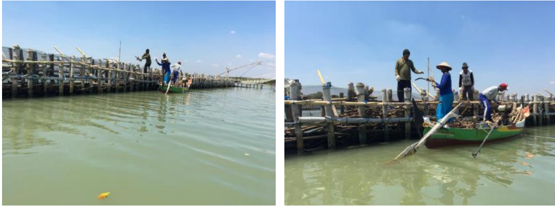
Figure 5.3: Permeable dams in Indonesia made with local labor and materials. Images kindly provided by prof. Susana Vinzón
