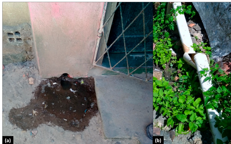
Figure 16. (a) Presence of water on the slope surface; (b) Damaged drain pipe.
