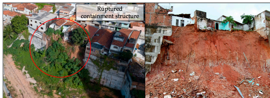
Figure 6. Area affected by the collapse of a retaining structure in the community of São José do Jacó.
