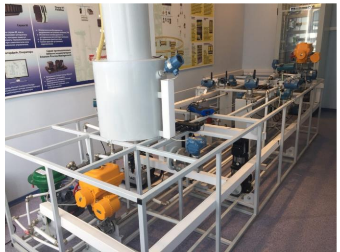
Fig. 7. Emerson flow test facility
